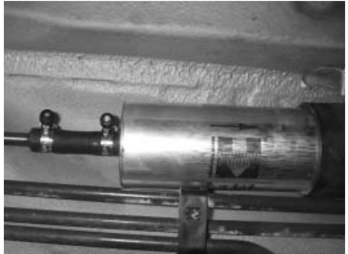
Photo #6 Inlet of new filter
