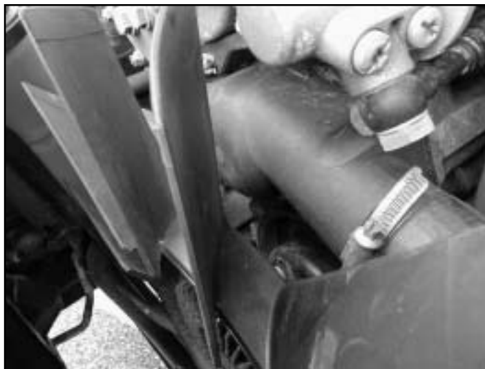
Photo 1: Old Housing Showing Deposits from Seepage.
